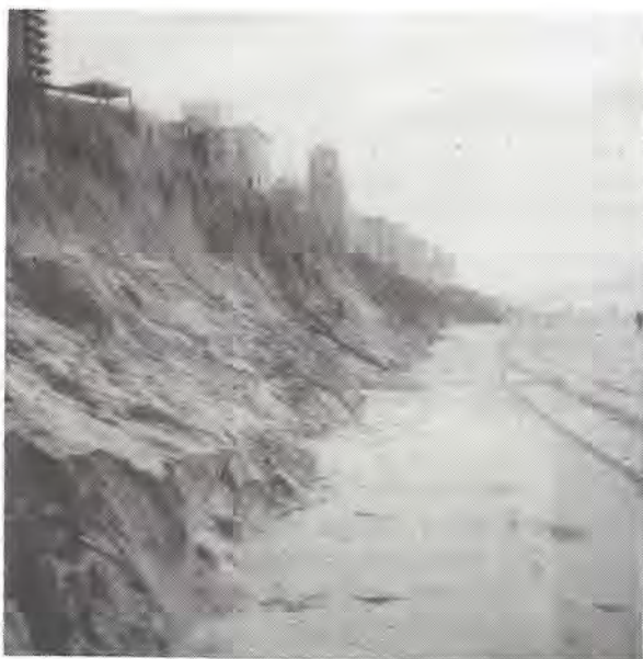
Fig 2.39: Eroding beach profile. Steep profile angle near dune area. Photo by Colin McMurtrie.
