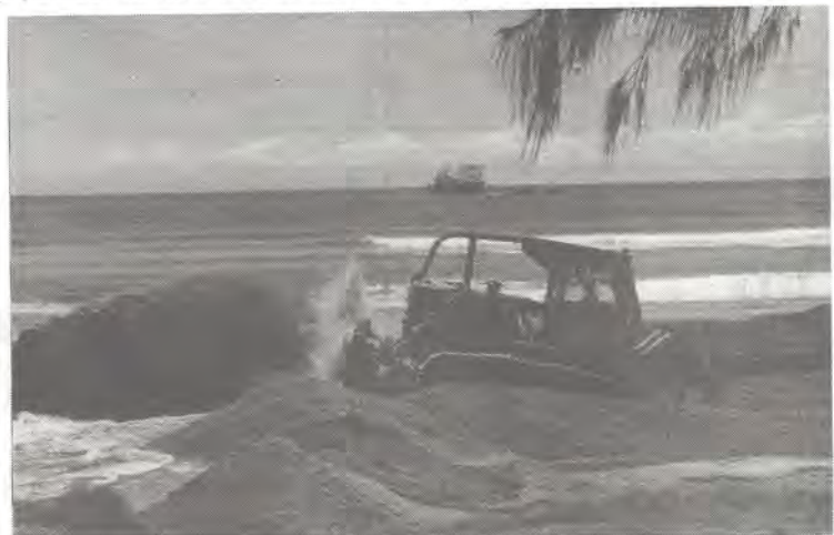
Fig 3.28: The pontoon was connected to a pipe to shore and sand gushed forth at a rate of 5,000 cubic metres an hour.
